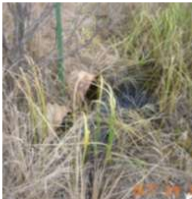
Figure 1 – Upstream End Unnamed Trib to Filson at Spruce Rd HW ~ 0.7 ft, but likely clogged
